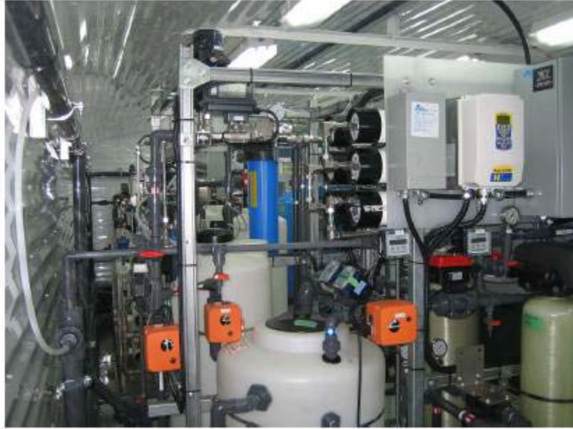
RO Units and chemicals
